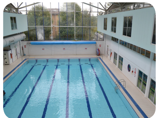
Main pool hall to have replacement LED light fittings
