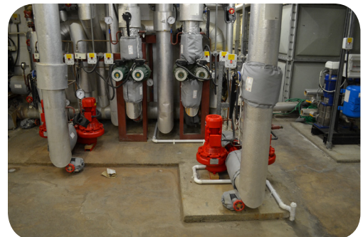
Variable speed drive motors to be fitted in plant room
