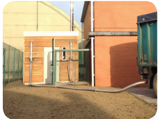
Wood pellets being delivered to new biomass boiler
